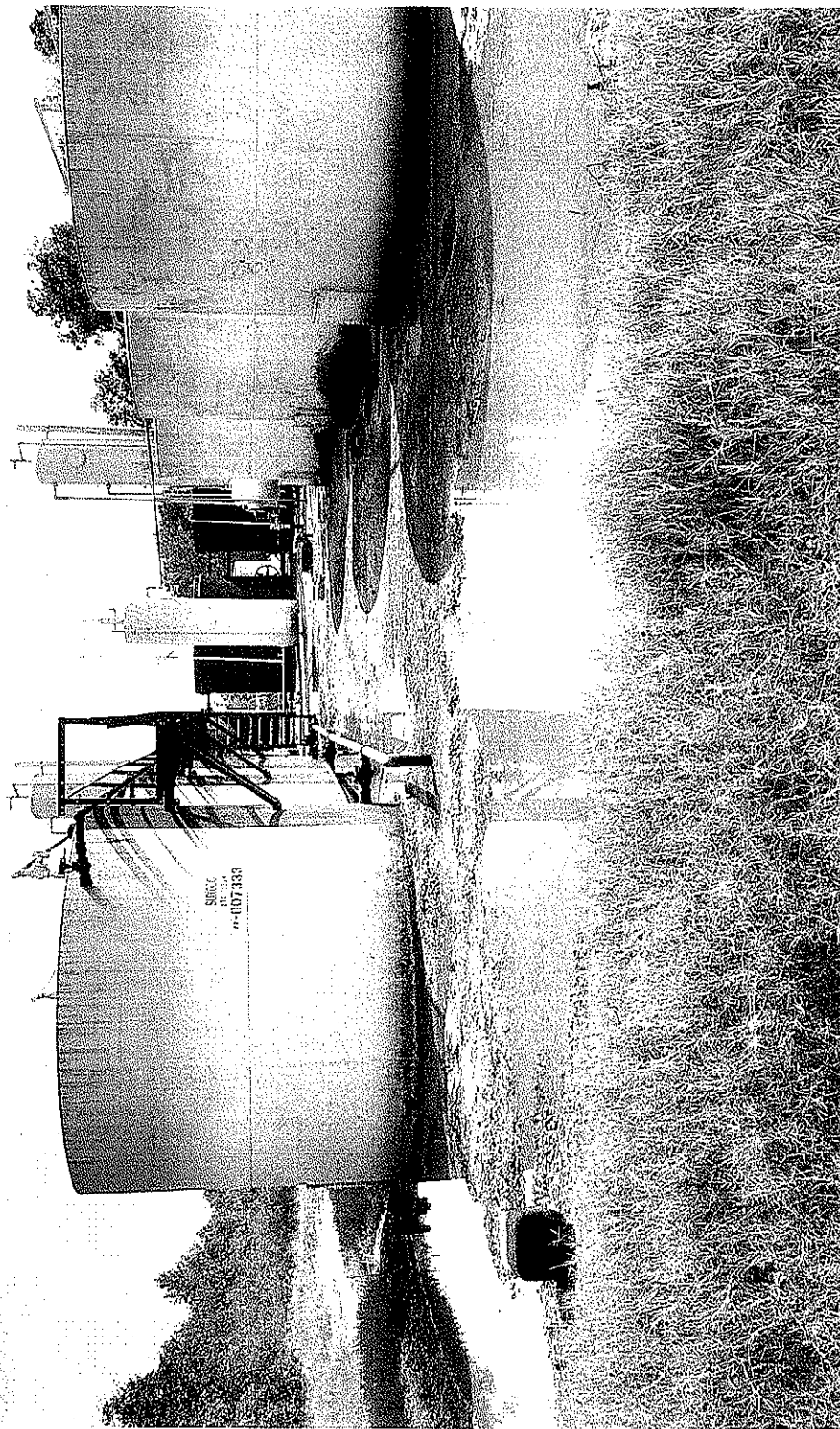
Photo 2 taken south. Brine pooled up inside tank battery. No rain here for weeks. 65k ppm TSS.
